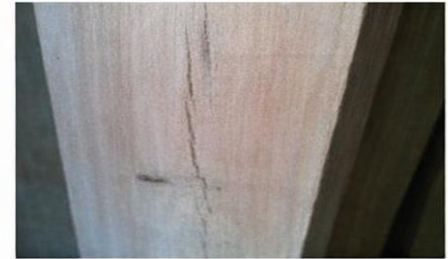
3. Cracks in Wood
